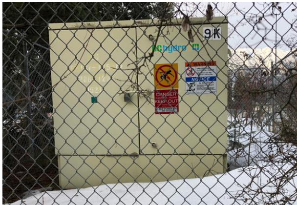
25kV:120/208V, 150kVA, 3PH/4W Transformer
