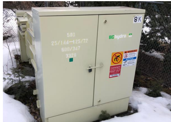
25kV:347/600V, 500kVA, 3PH/4W Transformer
